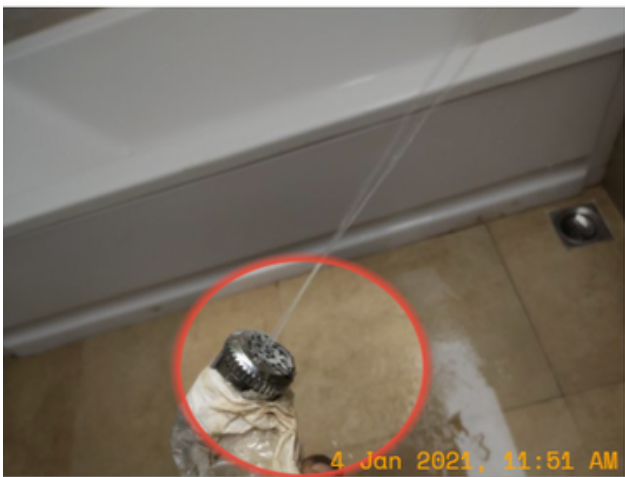
Health faucet gun holes blocked.
